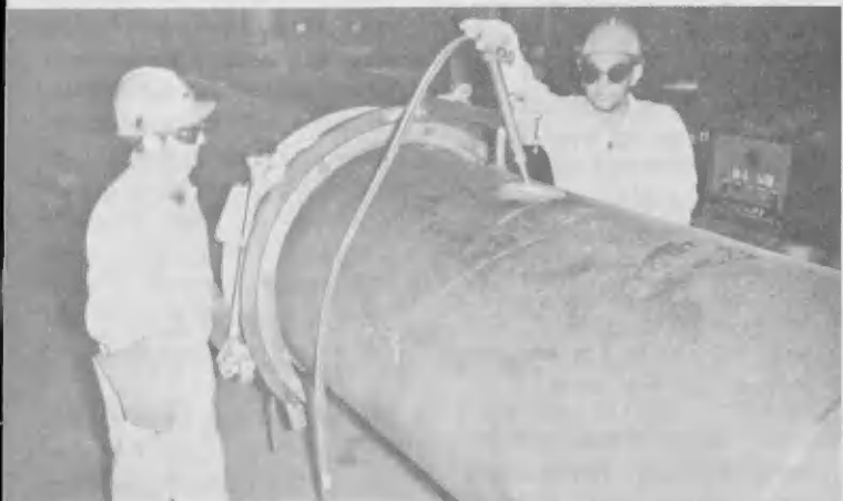
Welders G. Tromp and M. Lopez (r) join two pipe lengths in Welding Shop to make 80 ft. long sections.
